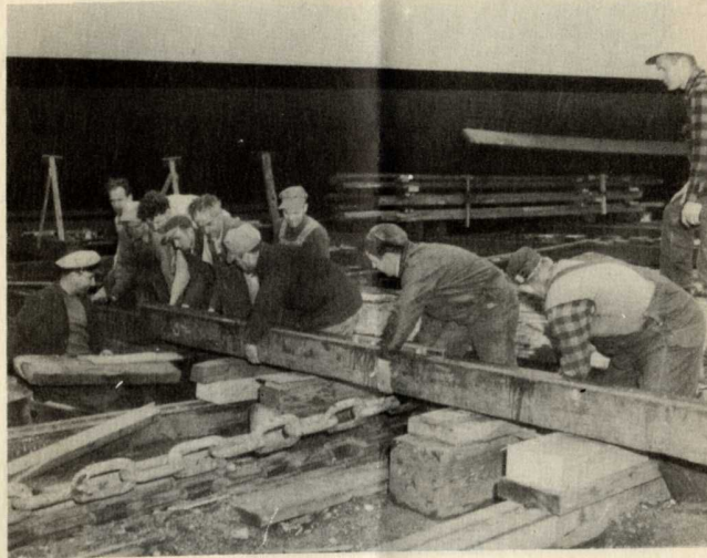
Hard at work on the ways, the Roustabout crew prepares for the next Minesweeper launching. For story, see page 1.
