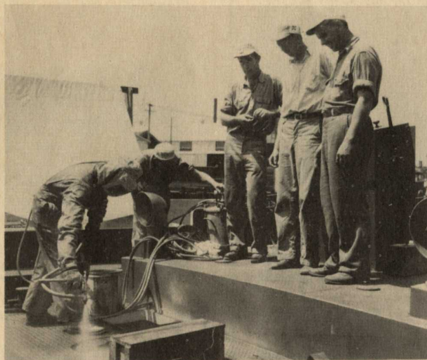
Employees of The G. R. & C. Paint Shop are shown at work on a steel landing craft. For story about "Buz" and the gang, see page 1.
